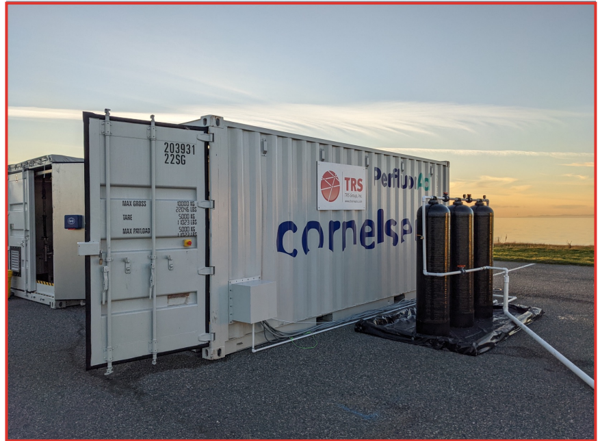
Continuous Flow (20 gpm) PerfluorAd Plant
